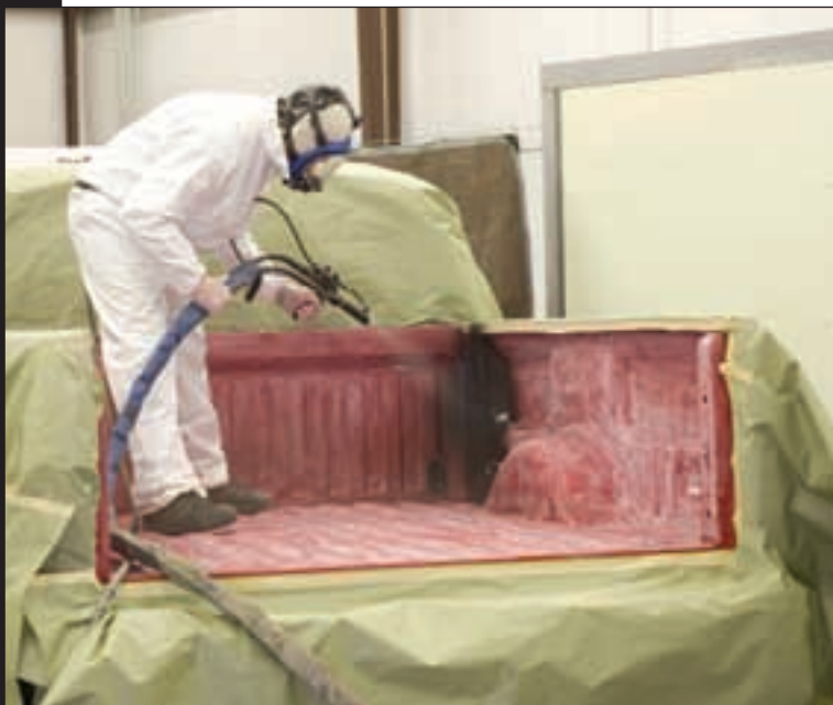
A flawless and efficient spray-on bedliner installation begins with a well-organized shop with adequate space.
